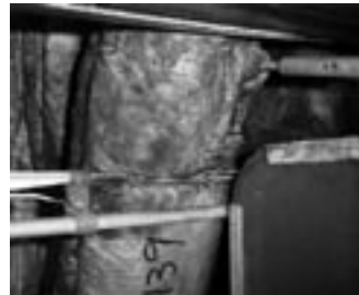
Corner of stowage bin (lower right) pushing the wiring into the insulation blanket and the underlying structural frame.
